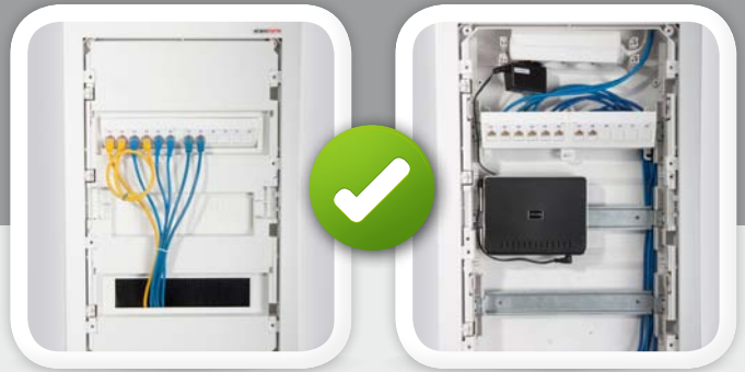
STAKOHOME-byT02 apartment data distribution cabinet
